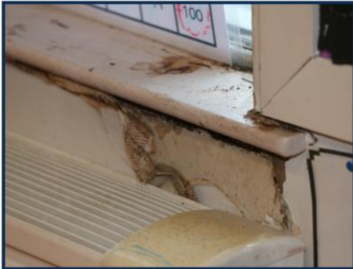
Internal damp and rot in classroom
