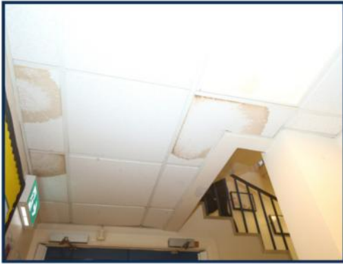
Damp on ceilings
