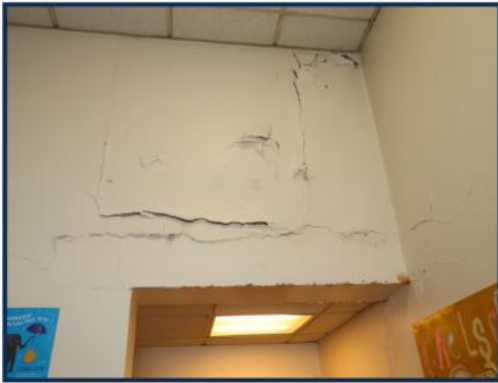
Damp on walls and ceilings
