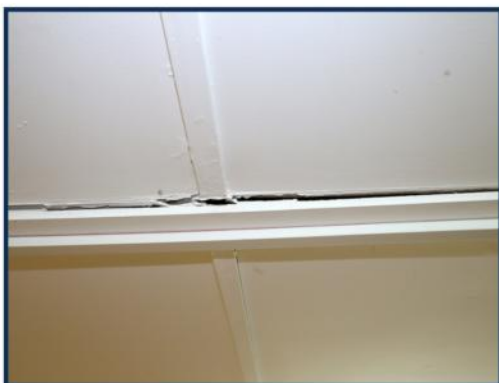
Damage to external classroom walls
