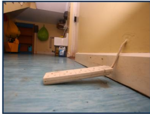
Health and safety hazard below main stairway
