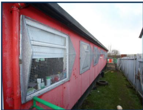
External paintwork in need of action
