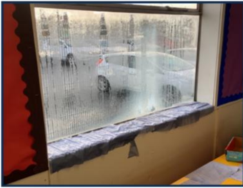
Internal damage during rainfall
