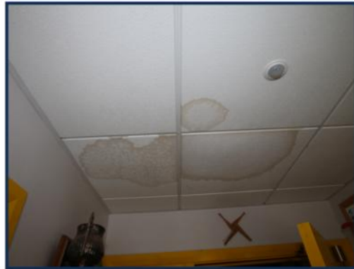
Damp on the ceiling of main school corridor
