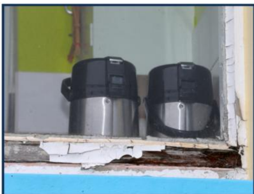
Close up of rot on school windows
