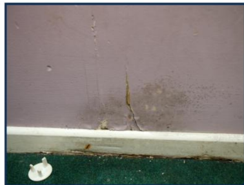
Dampness on internal walls of classroom
