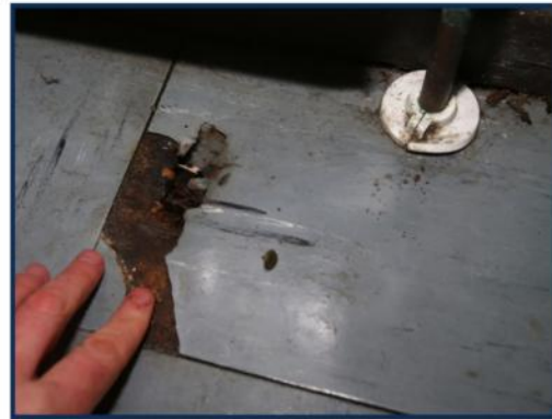
Rot on the floor of classroom
