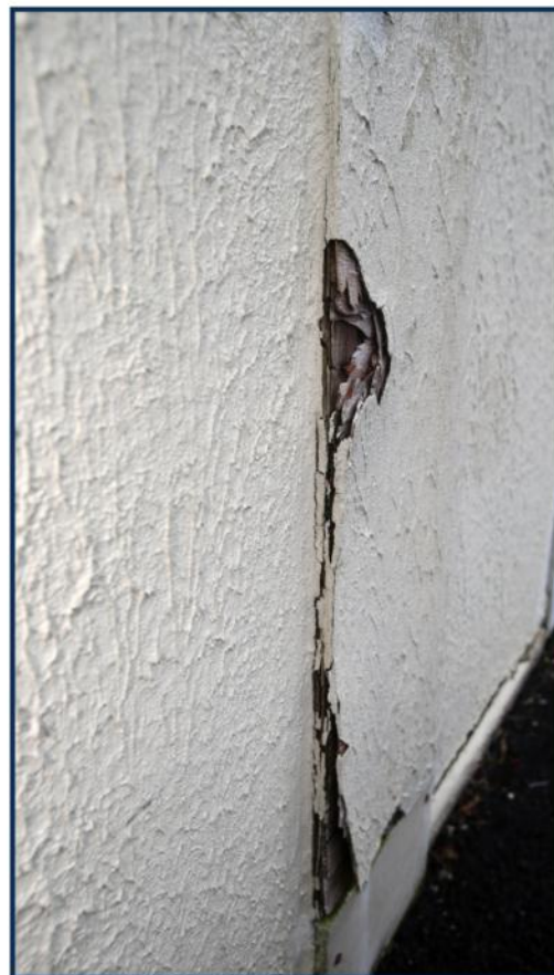
Close up of external rot
