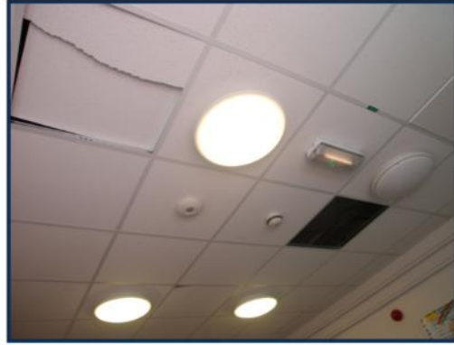
Damage to internal classroom ceilings
