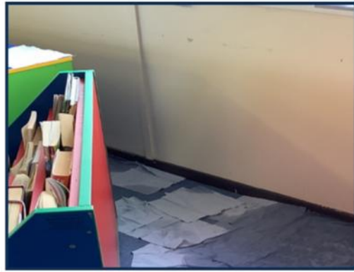
Flood in classroom during rainfall
