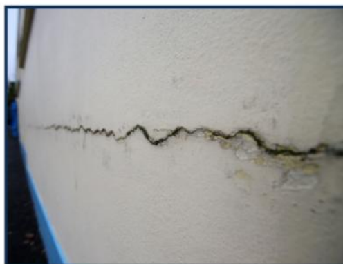
External rot on classroom walls
