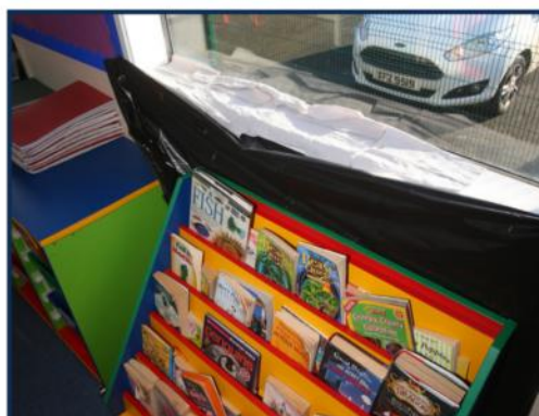
Damaged window with constant leak during rain
