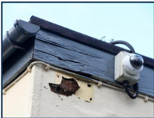
Rot to external walls of classrooms
