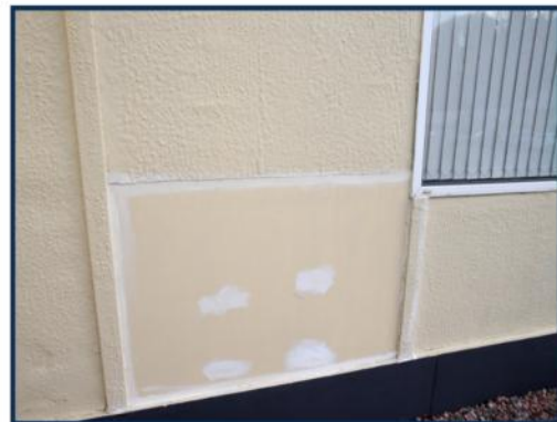
Patched paintwork on external classroom walls
