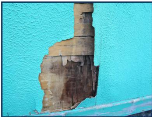
External rot of classroom walls
