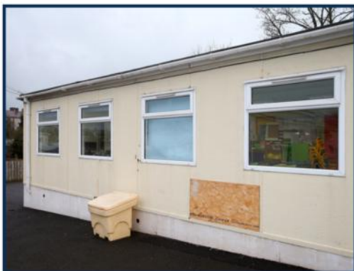
Damage and rot to all external classroom walls
