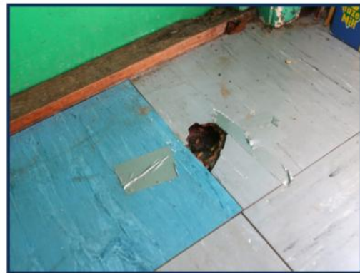
Hole in the floor of classroom
