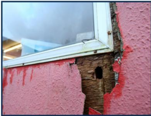
External rot of classroom walls
