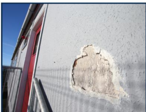
Damage to external walls of classrooms
