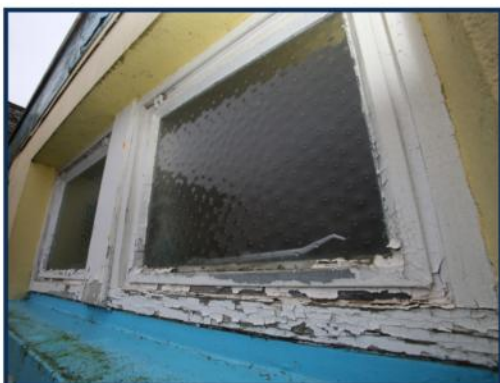
External rot on classroom windows
